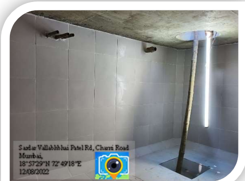
Underground water Tanks
