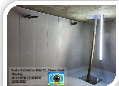
Underground water Tanks
